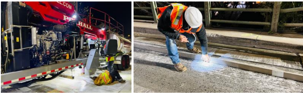
Figure 5: Diamond Grinding of the New PCC Validation of Smoothness Using a 16-ft Straight Edge
